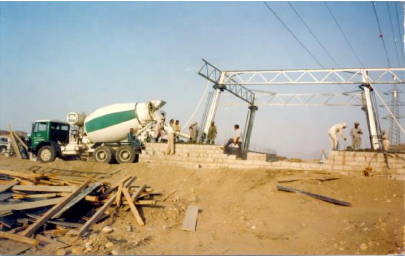
DIVERSION OF 110kV DOUBLE CIRCUIT O.H. TRANSMISSION LINES AT ARAFAT - MAKKAH (1992) Special Foundation Design on Solid Rock without excavation, Uplift and Compression compensated by RCC and PCC concrete volume of 637m 3
