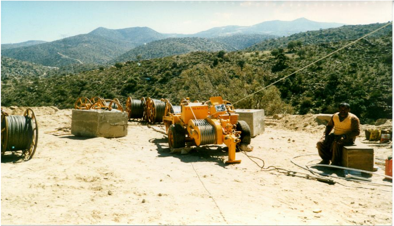
STRINGING OF 132KV DOUBLE CIRCUIT OVERHEAD TRANSMISSION LINES AL-BAHA (SUADIA) Stringing Activities in Progress at Puller / Tensioner Stations in one of the most difficult hilly terrain of the Southern Region of Saudi Arabia (1989) - By GEM SEEROO
