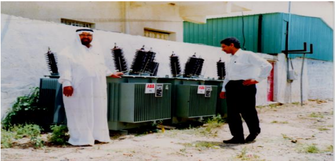
34.5kV Distribution Network Development System At Wadi Al Toraba, Southern Region of Kingdom of Saudi Arabia
